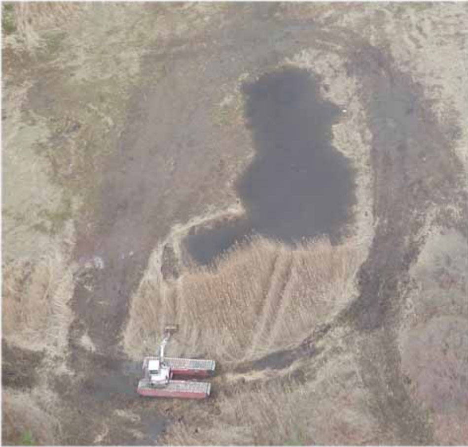
LEFT: Construction begins for one of the new ponds created in the Lower Connecticut River tidal marsh complex.
