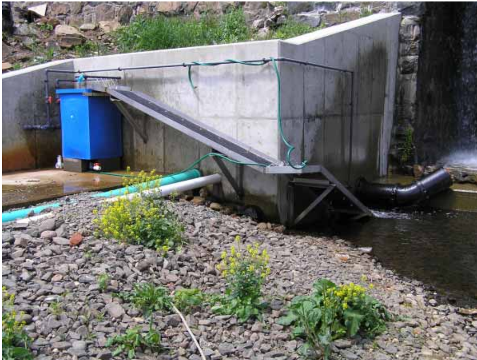
A view of the Mill River Eel Pass installed at the base of the Lake Whitney Dam in Hamden, CT.
