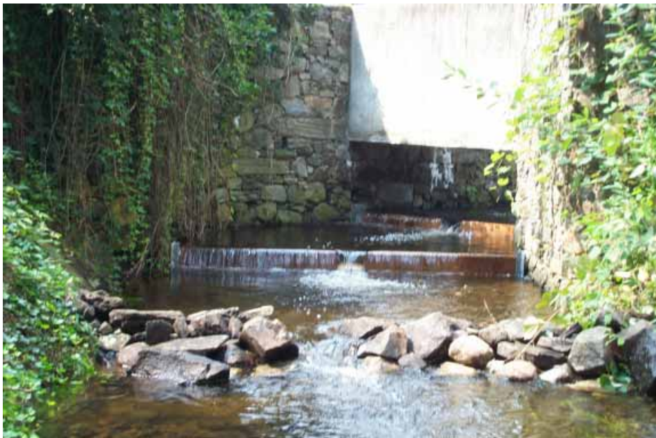
This pool and weir fishway allows migratory fish to bypass Dorr's Millpond Dam in the Saugatuck River.
