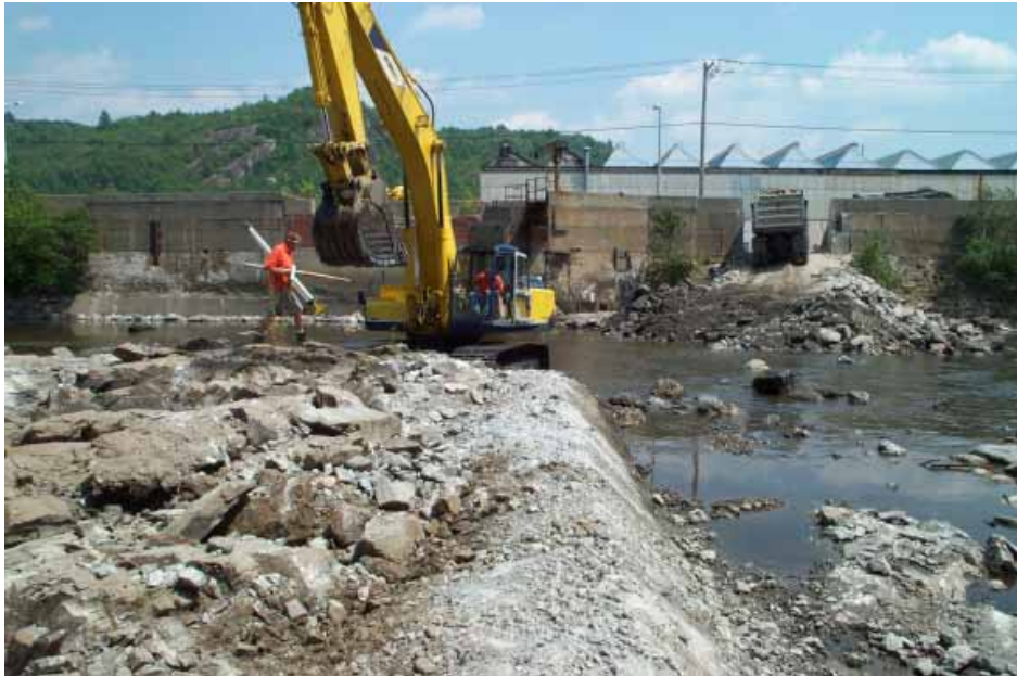
The Chase Brass Mill Dam was removed by the City of Waterbury as part of a legal settlement related to the Sewage Treatment Plan project.
