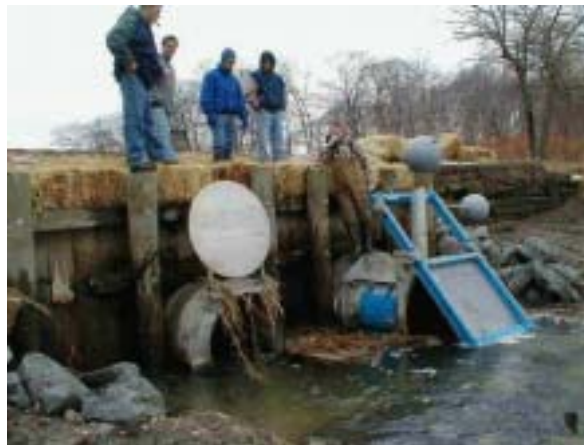
The pipe on the right is a self-regulating tide gate, the pipe on the left is a flapper gate.
