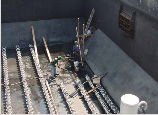
Jeanette Brown, opposite page, in front of one of Stamford's new biological tanks. Construction workers, left, cut a hole in cement between two tanks at the Stamford treatment plant.
