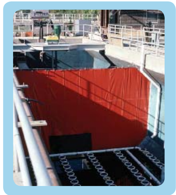
West Haven Sewage Treatment Plant 1996 upgrade. Anoxic Zone nitrogen removal tank. Photo by Gary Johnson, CTDEP.
