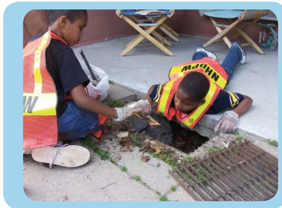
Stewards Juan Figueroa and Algon Dill cleaning out a storm drain behind their building run by Mutual Housing of South Central Connecticut. Photo by Hanifa Washington.
