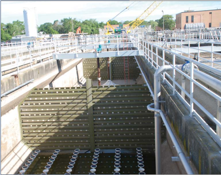
Figure 1. Stratford aeration tank.
