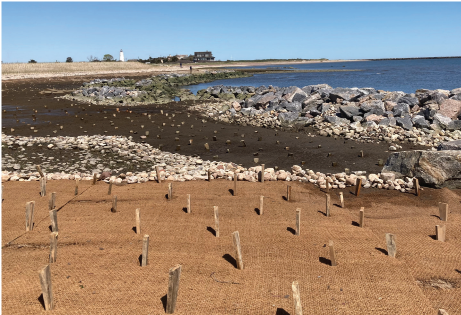
Looking east nearing project completion. Rock sills with cobblestone are centered between the restored dune planted with American beachgrass (background, left) and tidal marsh restoration site in the foreground, which was planted with smooth cordgrass shortly afterwards.
