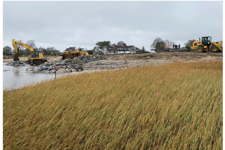
Photo looking west with dune (right) and living shoreline under construction. Existing healthy saltmarsh can be seen in the foreground.
