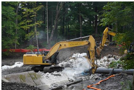
Dana Dam being demolished in Wilton, CT. The dam removal will enable migratory fish to reconnect with 10 miles of upstream habitat. Photo from Save the Sound
